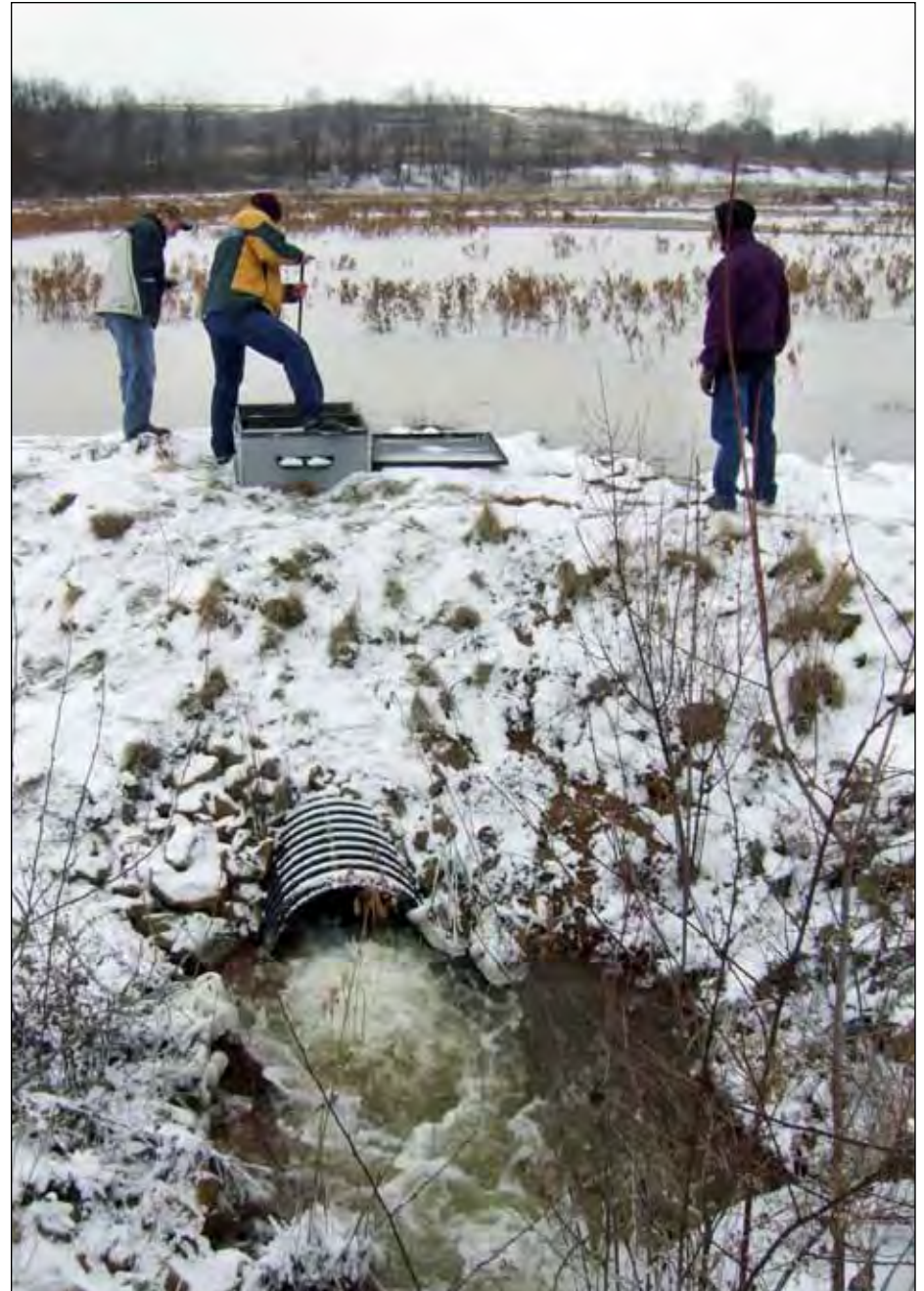
Adjusting the final flow control box where treated mine water from the Brinkerton Treatment System enters the Sewickley Creek in Westmoreland County.
